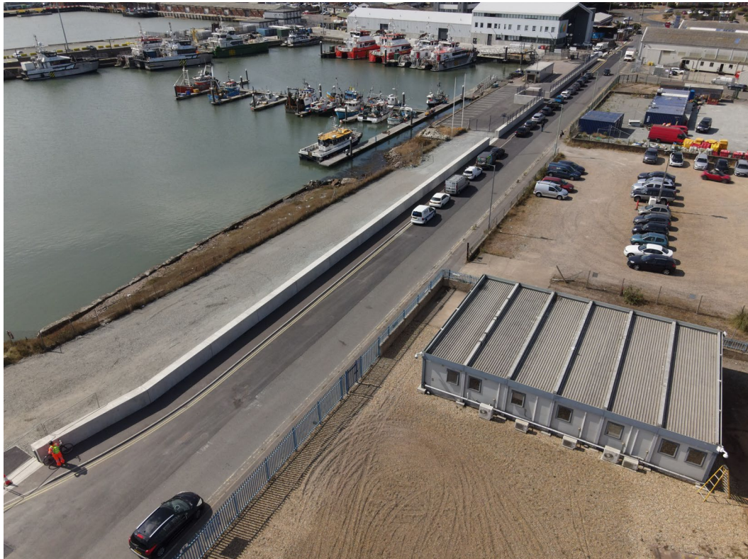
Lowestoft Flood Risk Management Project – construction of tidal flood walls, Hamilton Road. Photo credit: Joshua Freemantle
