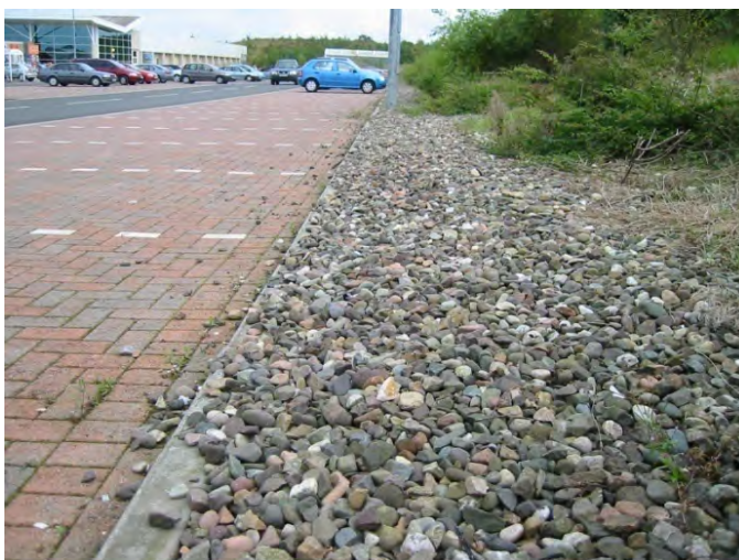
Figure 4b: Permeable paving
