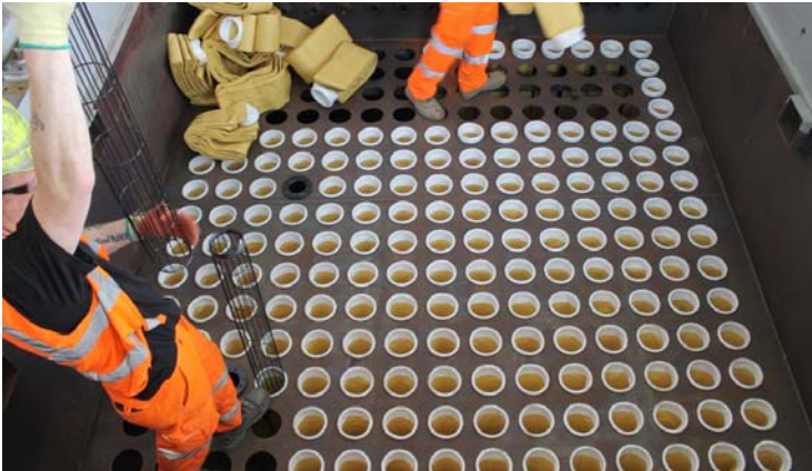
Flue gas filters (socks)
