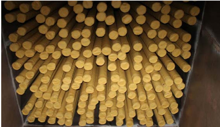
Flue gas filters (socks)
