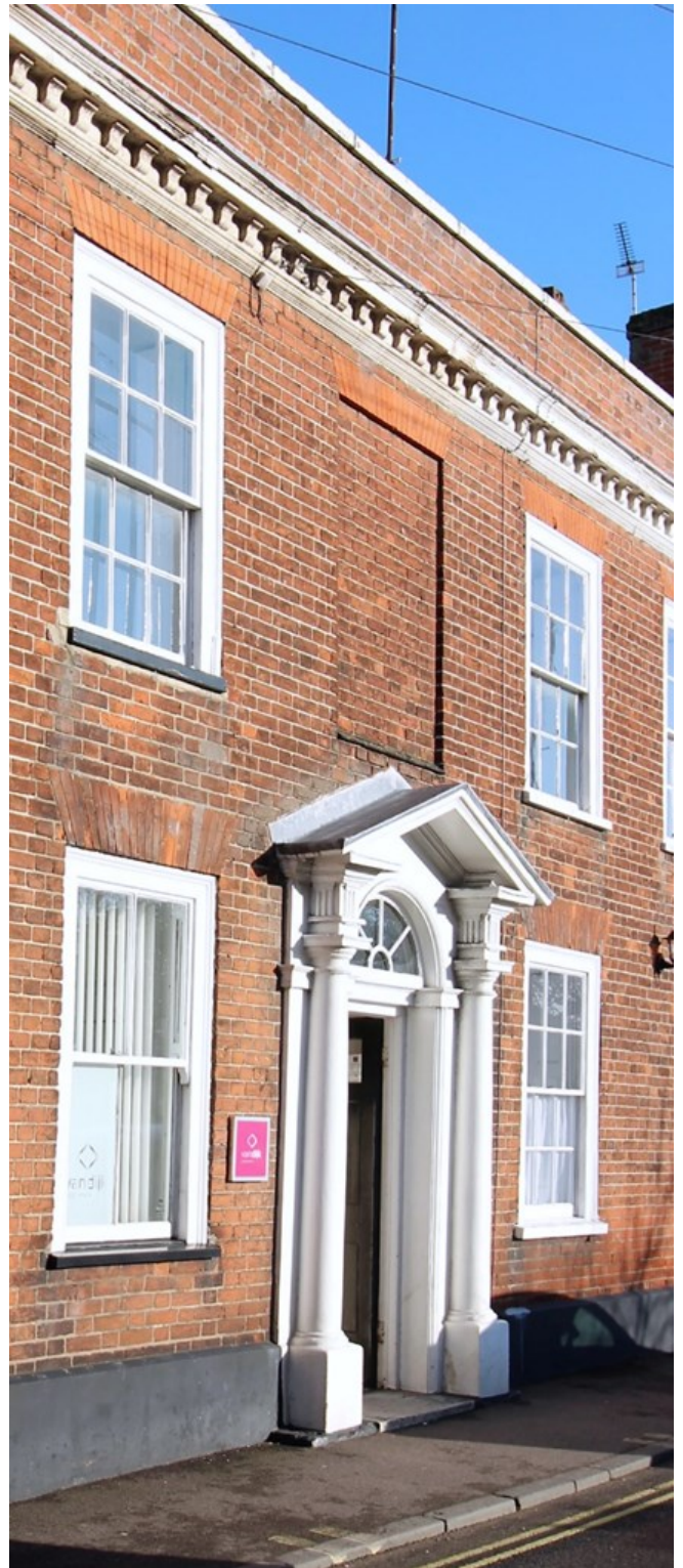
Left: Welsh slate roof on the early nineteenth century No.1 Broad Street
