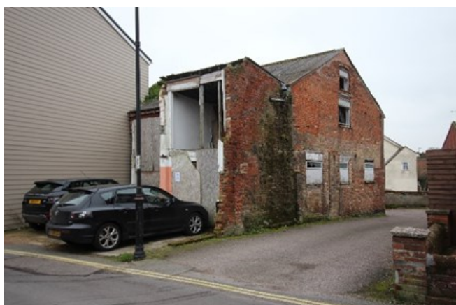
Poorly maintained warehouse Priory Lane
