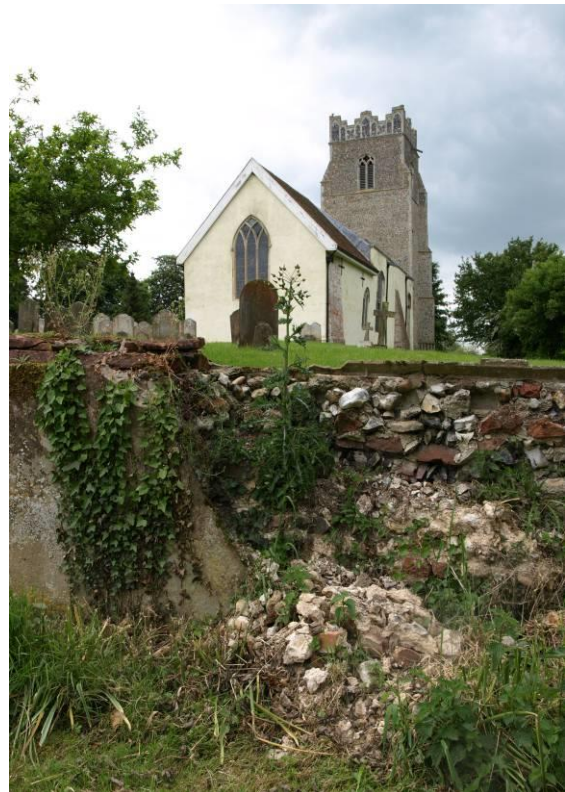
Damage to Churchyard Wall
