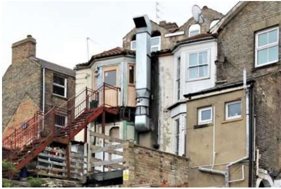
Poor quality conversion work to properties on the eastern side of High Street visible from Rants Score.
