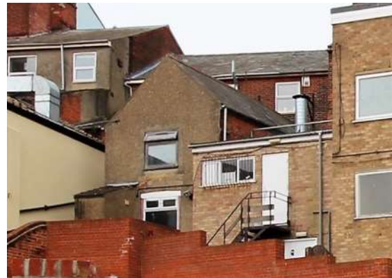
Rear elevation Nos.94-96 High Street with large twentieth century rendered range projecting to far left.
