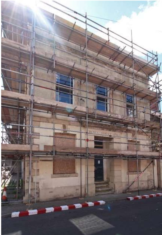
Crown Street Hall, Crown Street West, undergoing restoration and conversion to apartments (2017 now completed)
