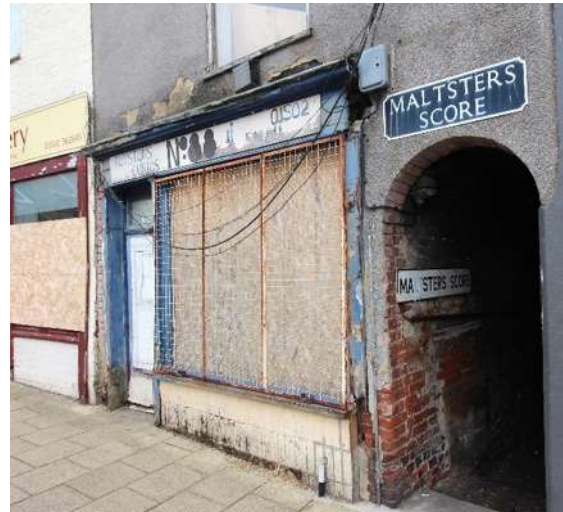
Derelict shops on the eastern side of High Street
