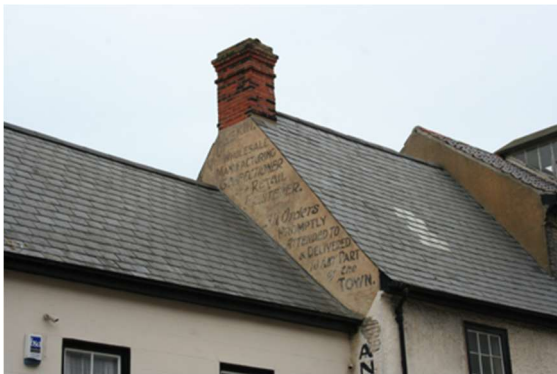
Remains of painted advertising sign to the gable end at No. 36 High Street
