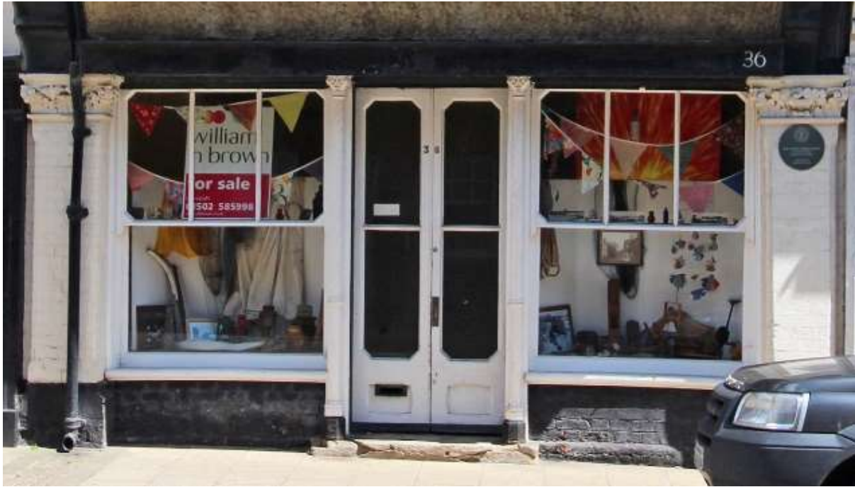
Detail of No.36 High Street. A late 19th-century shopfront with cast-iron columns set below the jetty of a 15 th century house
