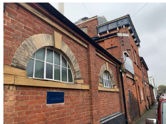
Detail of the brickwork to the Crown Brush Factory, Crown Street West
