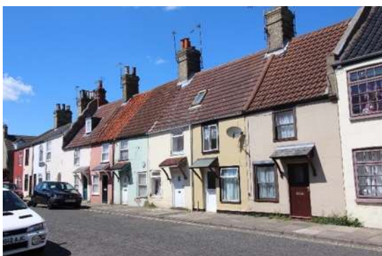
Listed eighteenth century cottages on St Margaret's Road the character of which has been harmed by poor quality replacement windows and doors.
