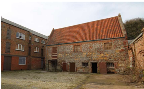
View of stone and brick elevation at the Fish House, to the rear of No.312-314 Whapload Road
