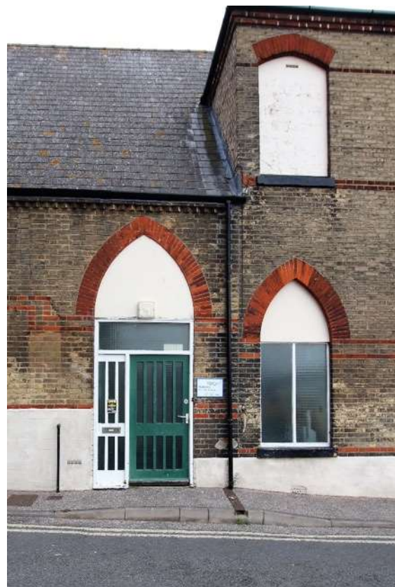
Poor quality replacement joinery, Herring Fishery Score
