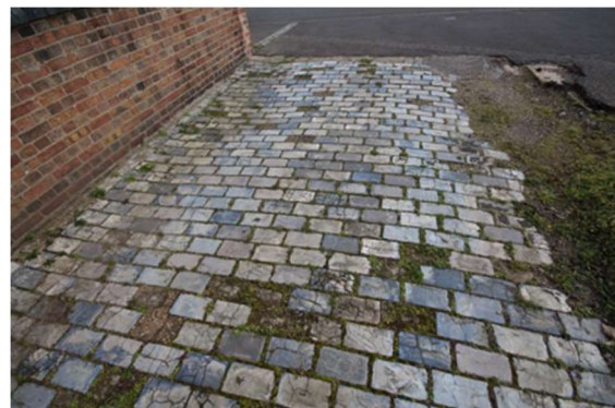
Stone setts, to the access track to the south of No.312 to 314 Whapload Road
