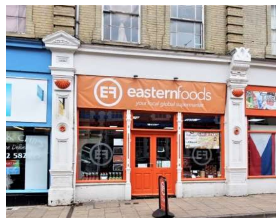
Detail of part of the frontage of the former Devereuxs Grocers and Wholesale Provisions Store. Designed by John Louth Clemence.
