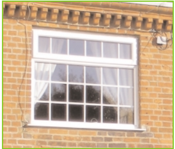
Poor design of replacement windows has a negative impact
