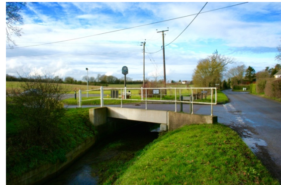
Figure 49: The negative impact of wires and their poles in key locations
