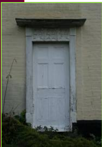
Fig 18. Example of one of the three seventeenth century timber doorcases at 60-63 High Street
