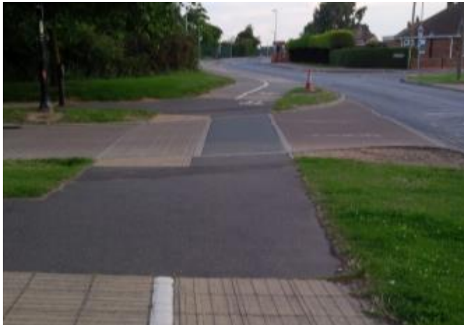
Cycle track crossing a side road. The use of surfacing and/or ground based cycle symbols can make it clear where cyclists should go once reaching the end of the segregated cycle track.
