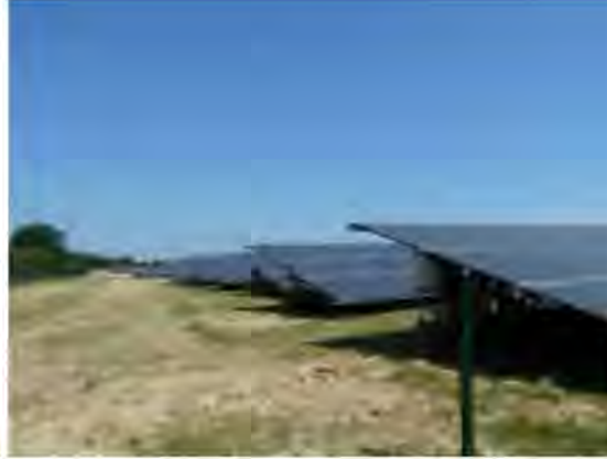
Photo 16: Solar farm, Ellough.
