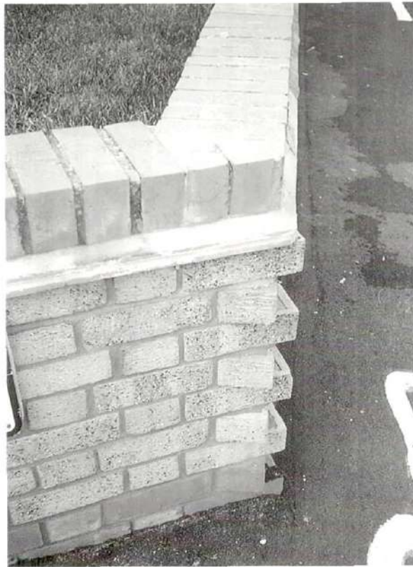
Poorly detailed angles . . .
