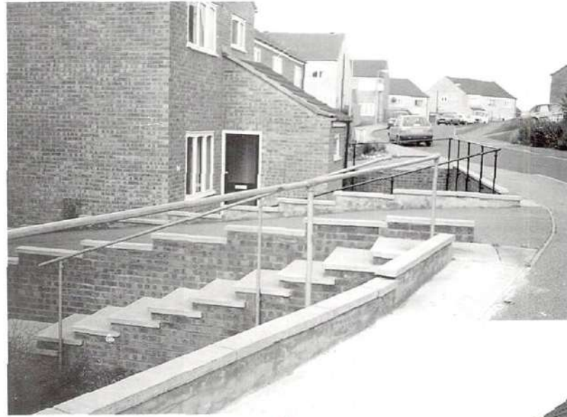
▲ Lack of attention to detail
