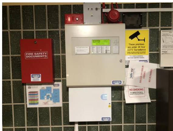
Control panel located in entrance lobby
